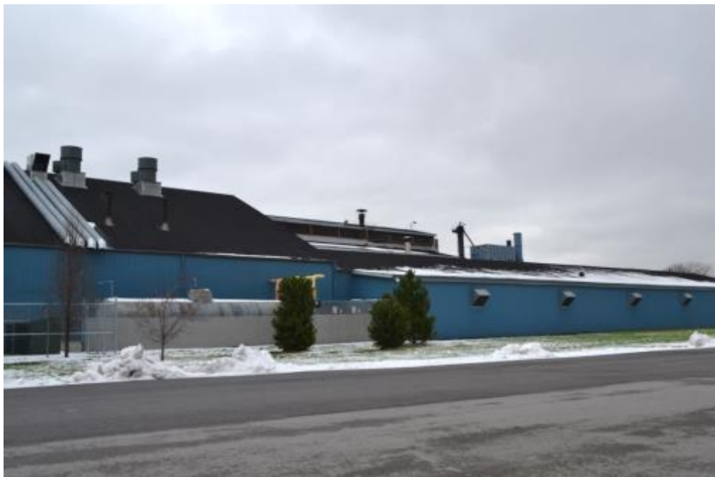
Figure 5-45: Sides of Original Buildings with New Corrugated Steel (view northeast)
